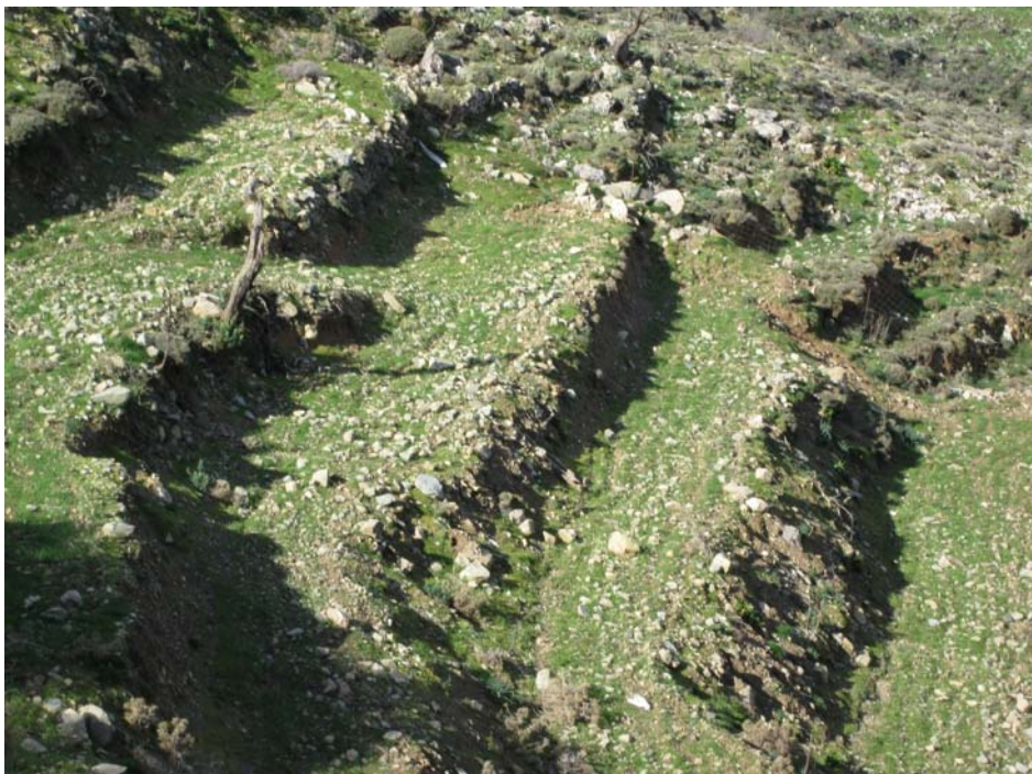
Fig. 2. Abandoned agricultural terraces in Crete, Greece. Lack of terrace maintenance combined with livestock grazing have caused failure of the terraces. Soil erosion and degradation leads to desertification of the land.
